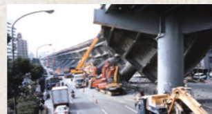
Sections of the Hanshin Expressway collapsed in the earthquake.
