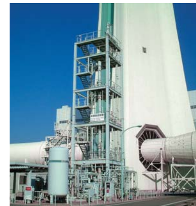
●Nanko Thermal Power Plant flue gas desulfurization plant
