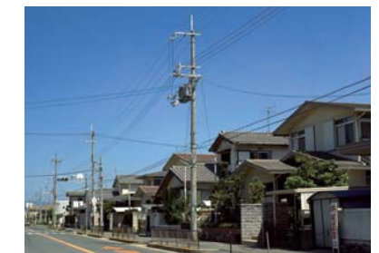
●Electrical pole and transformer
