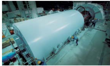
● Combined cycle electric power facility (Sakaiko Power Plant)
