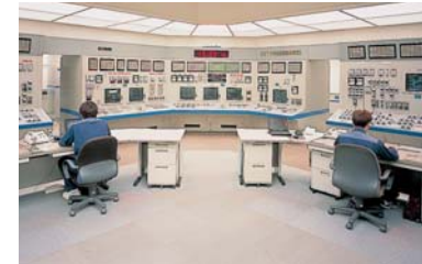
● The Central Control Room in a nuclear power plant
