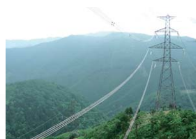
●Power transmission lines
