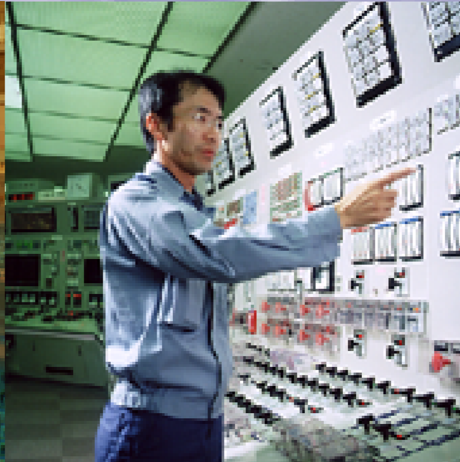
Central Control Room (Takahama Nuclear Plant)
