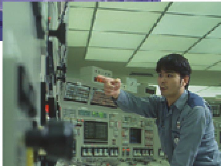
Central Control Room (Takahama Nuclear Plant)
