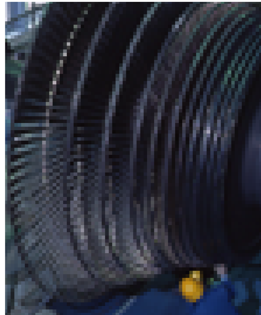
Low-pressure turbine inspection
