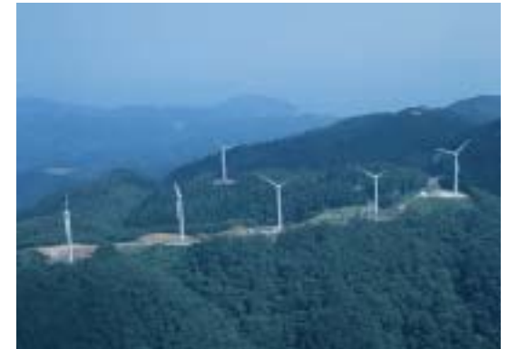
Wind-power generation equipment supported by Kansai Green Power Fund (Taiko-yama, Kyoto)
