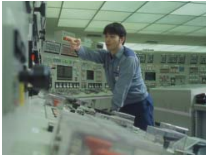
Central Control Room (Takahama Nuclear Plant)
