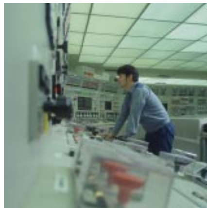
Central Control Room (Takahama Nuclear Plant)
